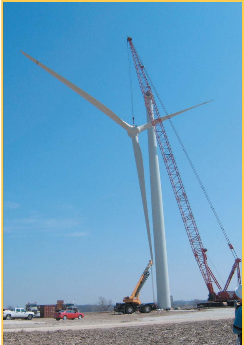
Many parts of the nation previously thought to lack wind resources can now generate wind power, thanks to advances in turbine technology. This turbine was recently erected by the Illinois Rural Electric Cooperative (IREC). Photo courtesy IREC
